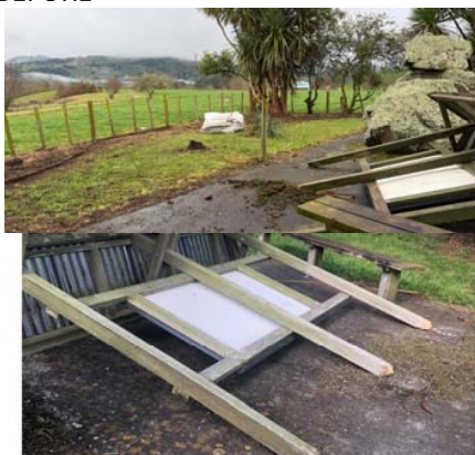
Photo: Damaged shelter due to heavy rain and high winds.
